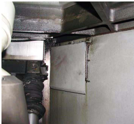
Figure 30 Deflector plate over extraction point
