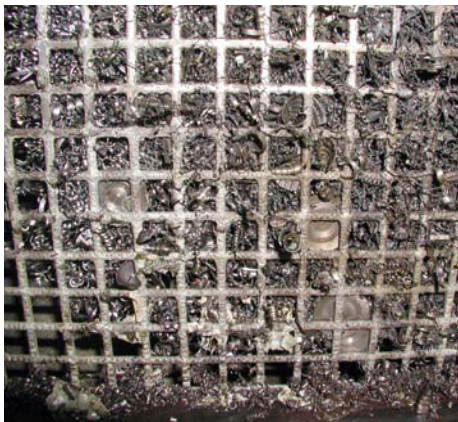
Figure 29 Clogged chip screen
