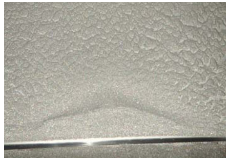
Figure 49 Caking on the panels
